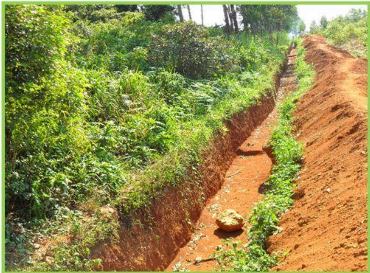
FOR THE PROPOSED CONSTRUCTION OF A 25 KM ELEPHANT TRENCH ALONG THE BOUNDARY OF KIBALE NATIONAL PARK
